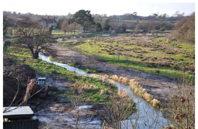
Removal of embanking along the river Glaven at Hunworth 2009, to help restore the river's connection with its floodplain.
